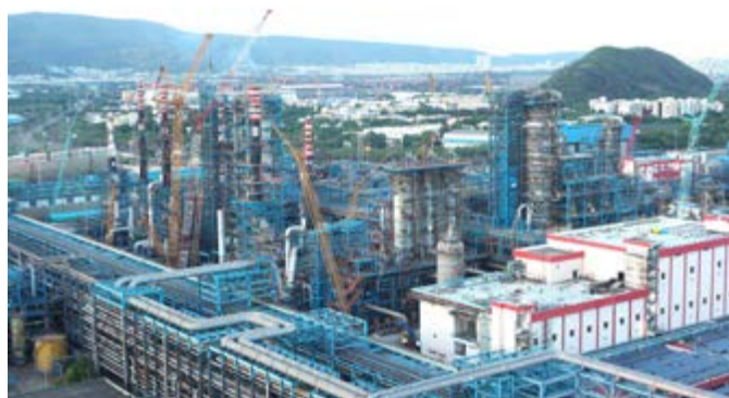
Residue Upgradation Unit (RUF) at VRMP
