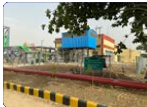
10 MW electrolyser based Green Hydrogen plant of 4.3 TPD
