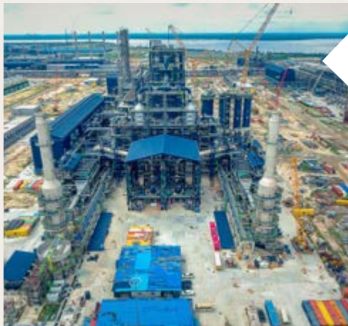
EIL signed contract with Dangote Oil Refining Company in 2014 to implement a 650,000 bpd refinery and an 830 KTPA polypropylene plant in Nigeria, the largest single-train refinery in the world.
