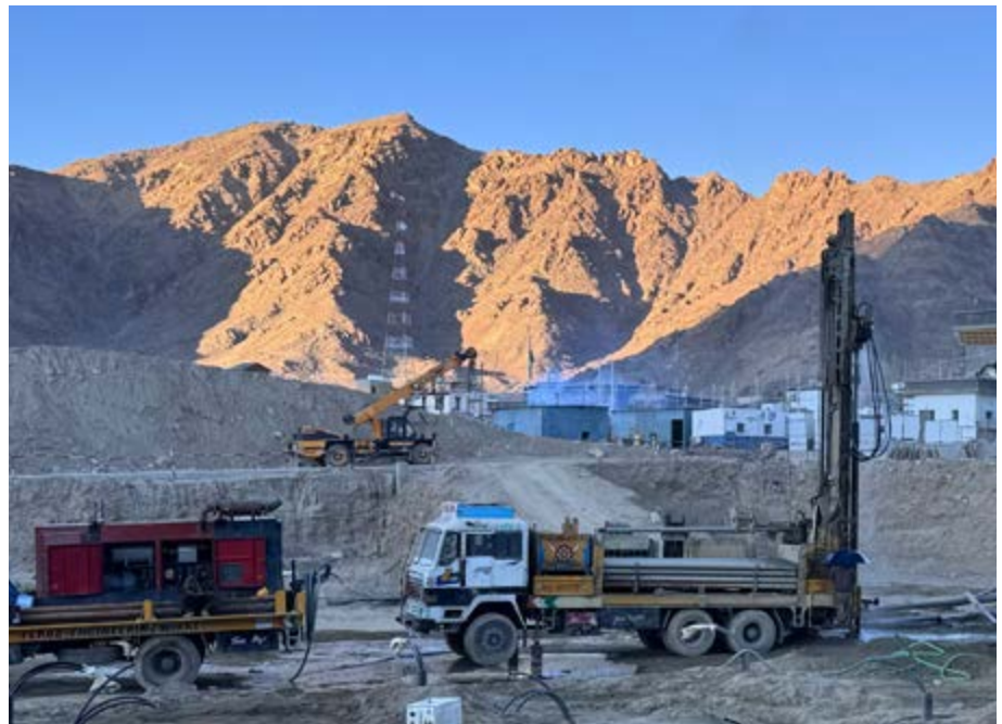
Application of Geo Thermal Engineering for Energy Management at Leh Airport
