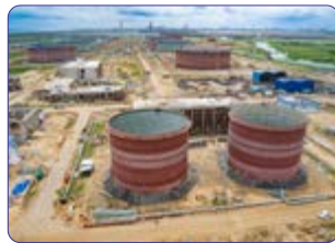
Crude Oil Terminal (COT) at Paradip, Paradip Numaligarh Crude Oil Pipeline (PNCPL)
